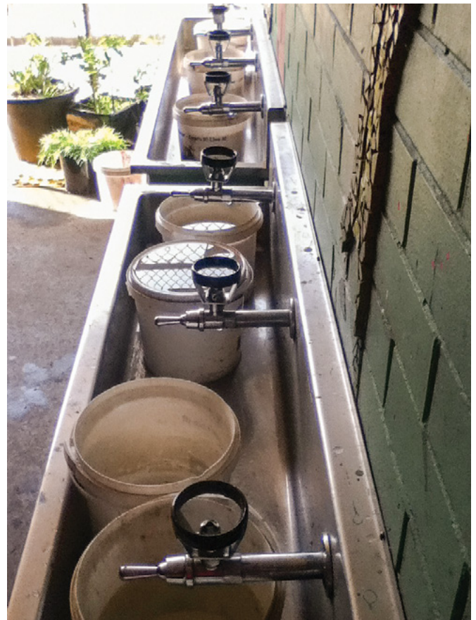
Manchester Primary School, Mooroolbark, using a simple solution for capturing and reusing water.
